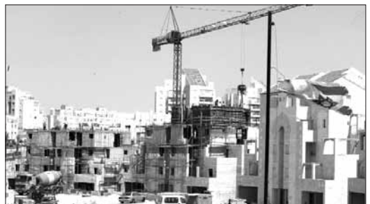
Workers build new buildings at the West Bank Jewish settlement of Maale Adumim, August 25. (AFP File Photo)
